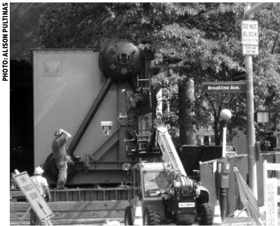
Following a final regulatory OK, workers began preparing the MATEP plant to receive a third turbine.
